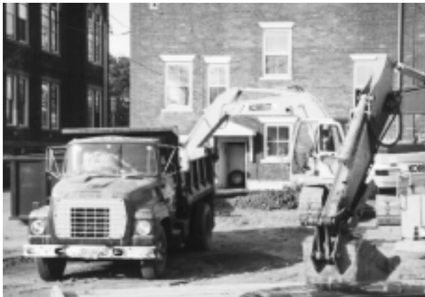
The "big dig" at the Masonic Hall involved carting away truckloads of brick from the interior demolition.
